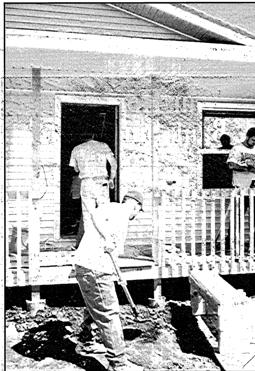
Workers put the finishing touches on the landscape of the McCoy home after the building portion of the project was completed.
